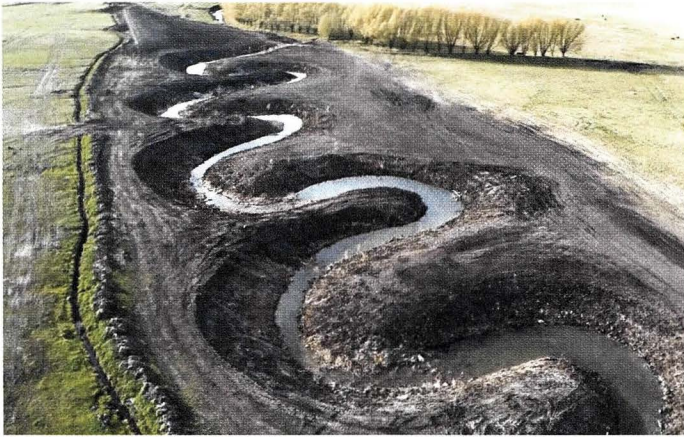
The Wallsburg conservation project restored natural meanders to this riverbed which reduced sediments flowing downstream into Deer Creek Reservoir.
